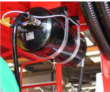
Tank with overpressure safety
